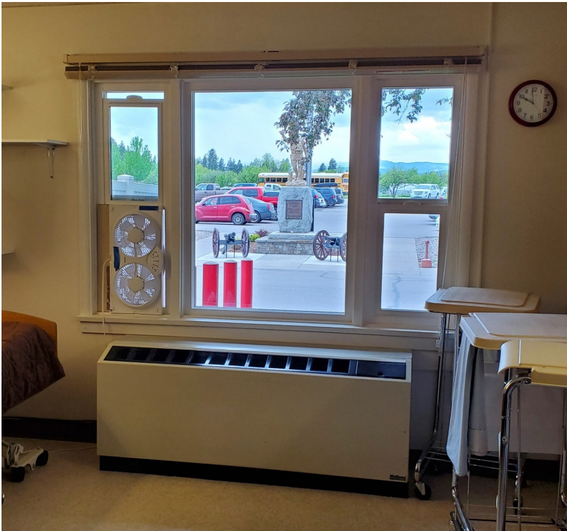
Typical Resident Room Hot-Water/ Chilled Water Fan Coil Unit
